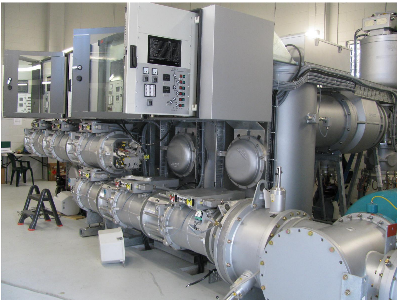
Figure 34: Sample gas insulated switchgear
