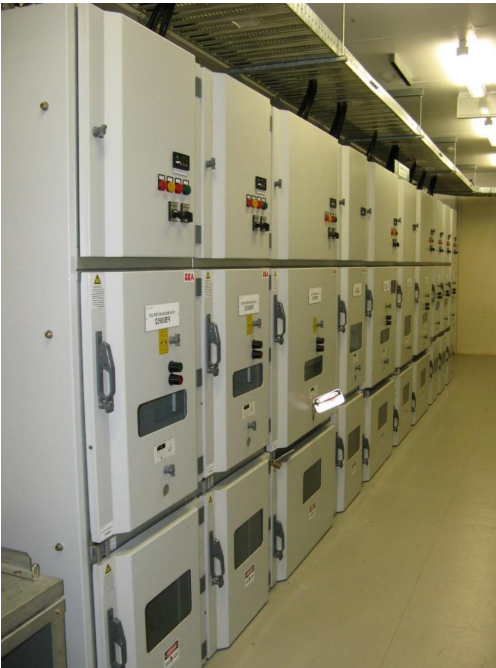
Figure 32: Sample withdrawable switchgear
