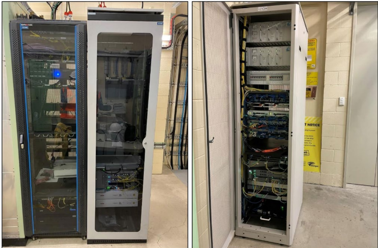
Figure 2 - Ciena rack doors (left) and MPLS door (right) – Beenleigh Substation
