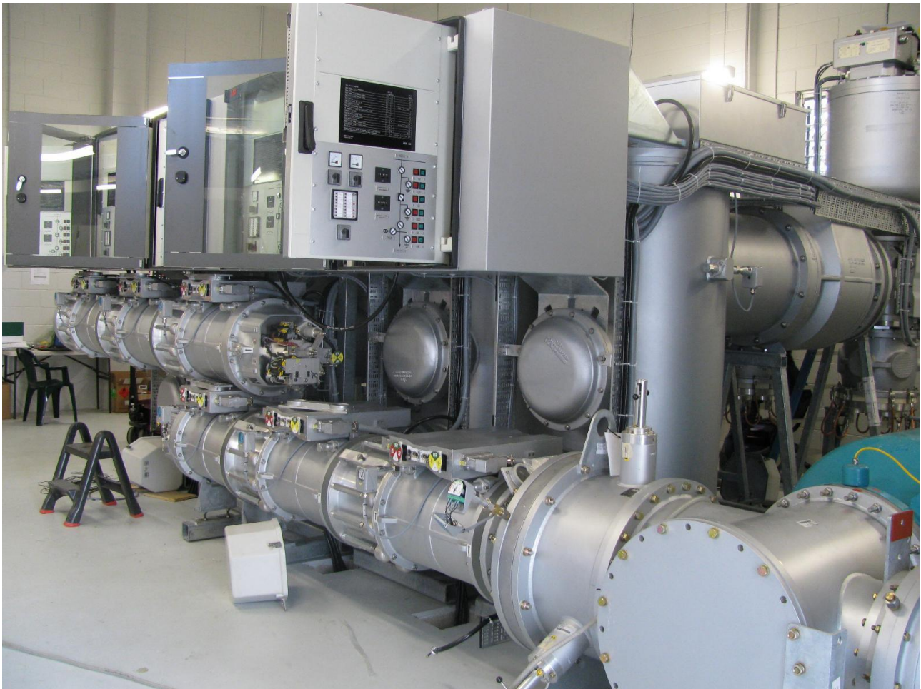
Figure 34: Sample gas insulated switchgear
