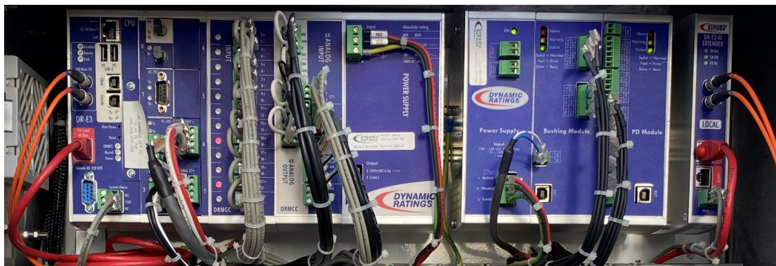
Figure 28: Example of brownfield DR-E3 at Barcaldine substation on transformer 2
